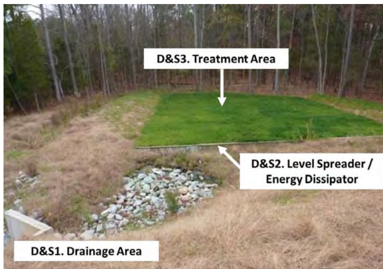
Figure 2.4.1 Key Areas for Level 1 Inspection of Disconnection and Sheetflow with filter strip shown.
