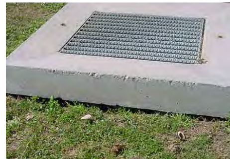
Water is “piping” down to the underdrain at the weak spot where the soil media meets the concrete overflow structure.
