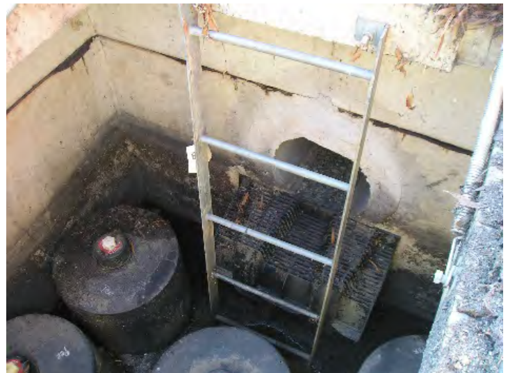
Figure 2.12.2. Examples of underground filters: Left –Perimeter sand filter in a concrete box (photo shows the filter with the grate top off as the filter is being maintained). The right-hand side is a sedimentation chamber filled with water and the left-hand side is the sand filter chamber. Right –Underground vault filter with special organic filter media inside cartridges.
